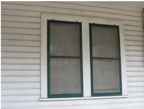
Like storm windows, screens may be fitted into original window openings (1207 St. John Street).
