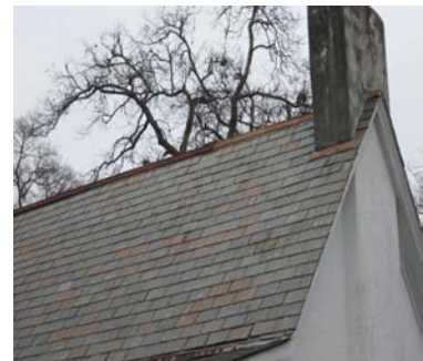
The slate roof at 1005 S. Grand Street is a unique historic elements that should be preserved. Maintenance is more cost effective than replacement in kind.
