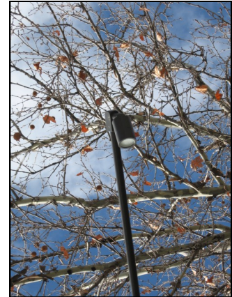
Above is an example of an appropriate exterior pole light .
