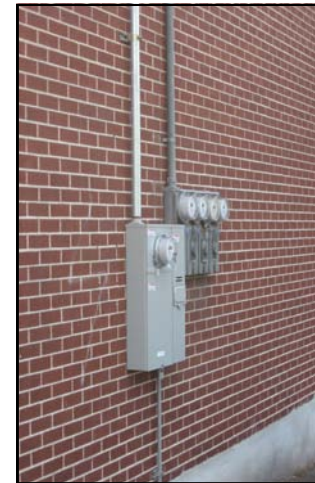
These meters are correctly placed on a non-primary elevation.
