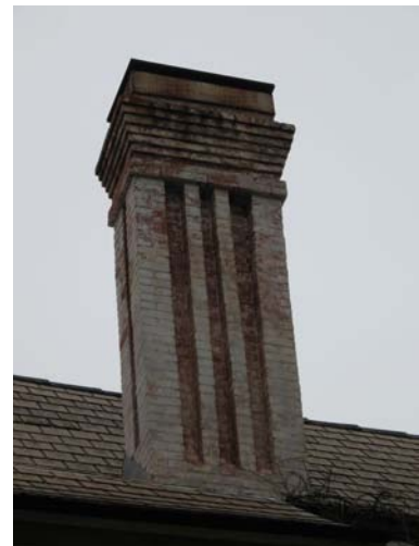
This detailed brick chimney at 918 Jackson Street should be maintained and preserved.
