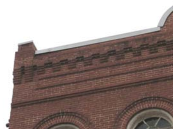
Preserve and maintain architectural details such as the corbelled brick cornice at 125 St. John Street.
