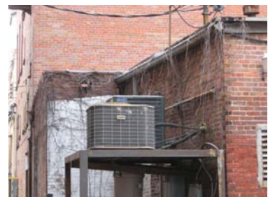
This HVAC system at 211 Desiard Street is situated on the rear elevation.
