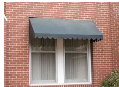
An awning, like this one at 201 Stubbs Avenue, should span the exact length of the opening it is to cover.
