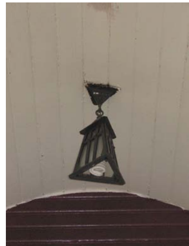
Over-head hanging light fixture at 406 Auburn Avenue.
