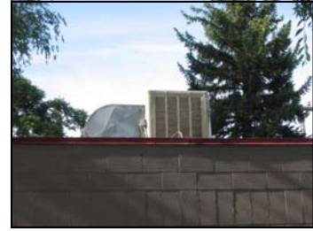
This roof mechanical system is set back so that it is not readily visible from the street.
