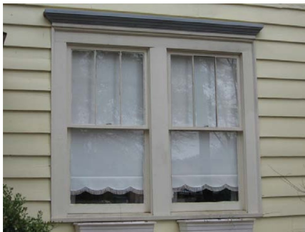
Original vertical-three-over-one wood sash windows help convey a dwelling's historic character. Replacing them would diminish the building's architectural integrity (100 Hudson Lane).
